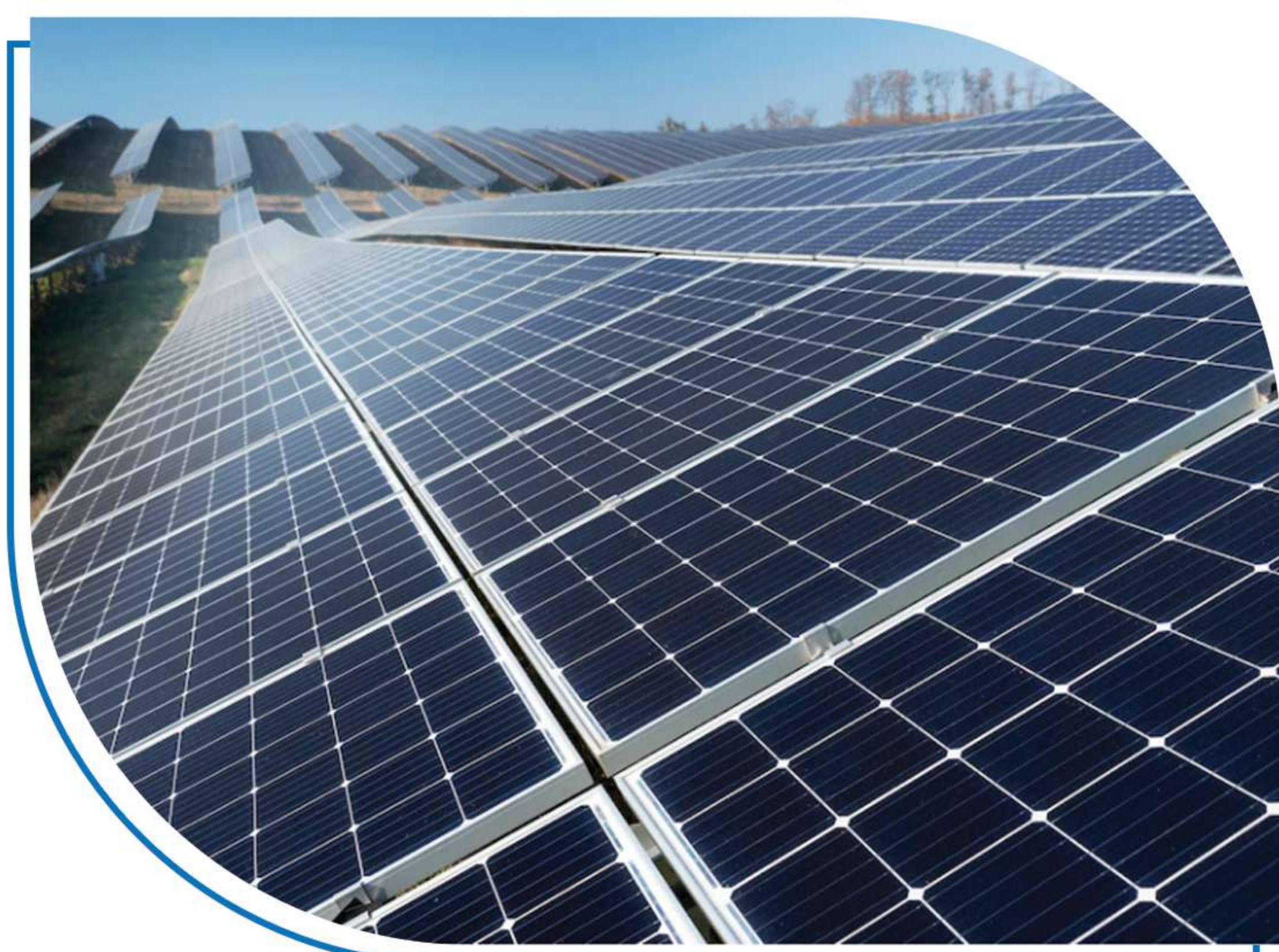
Solar Panel Structure
